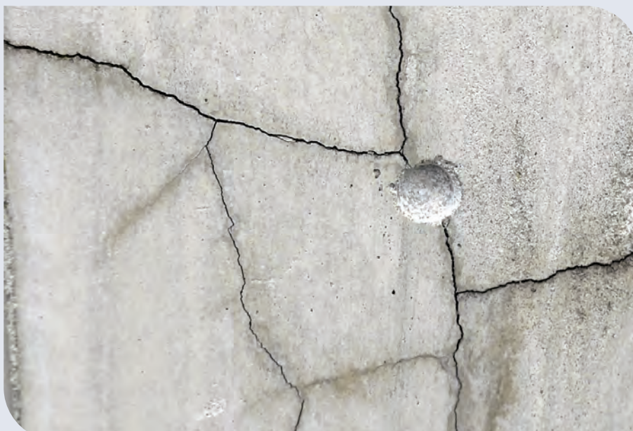
ABOVE: Cracking in over-thick or non-compatible facing coat.
